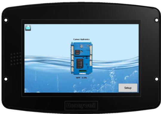
Figure 27: Control Panel Front
